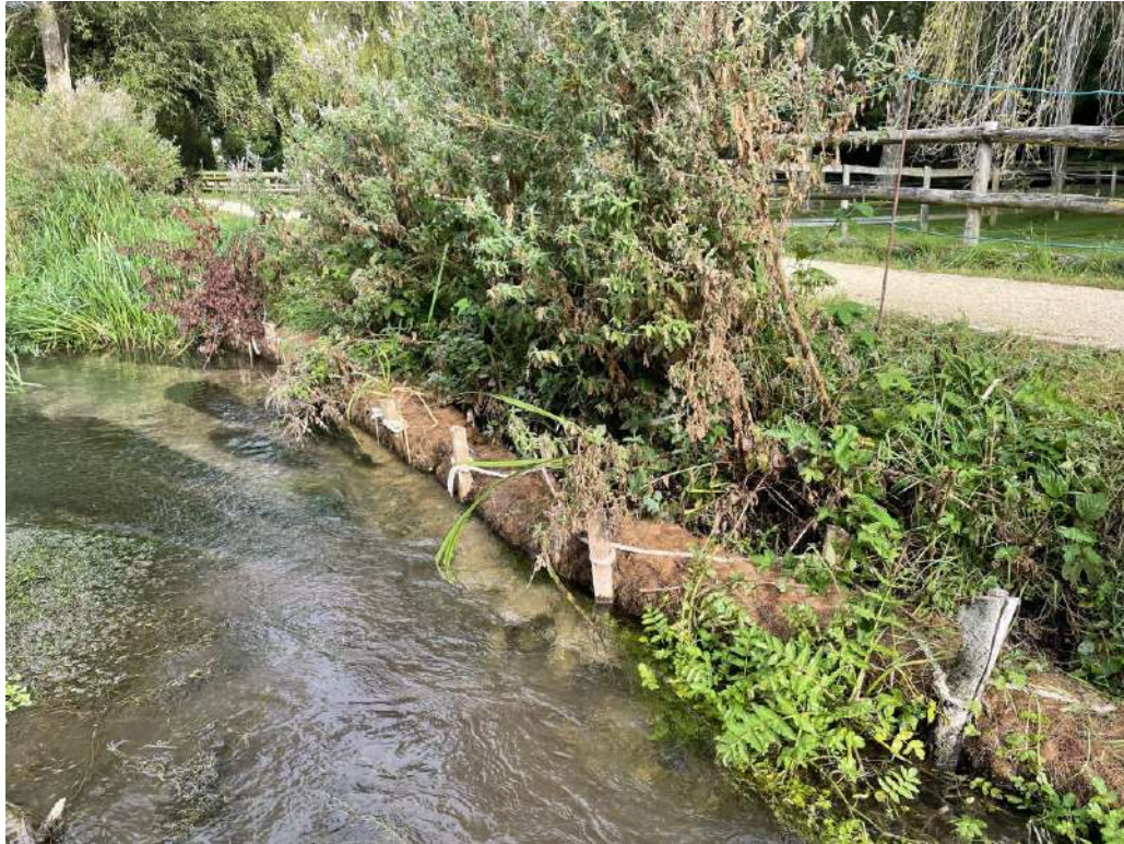
Restored section of bank showing coir fibre roll; vegetation on the roll has established well in some places but not in others
