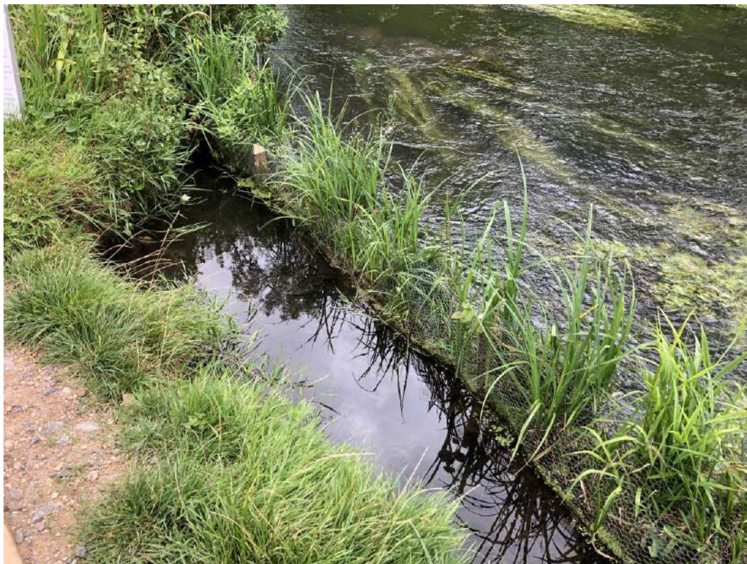
Coir fibre rolls installed in Section 6 where displacement took place; vegetation still establishing
