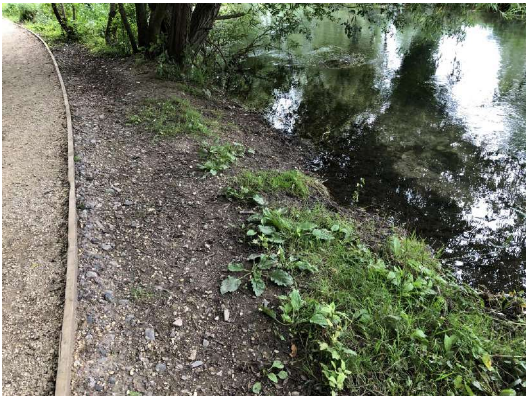
Section 4 – area of damage to bank
