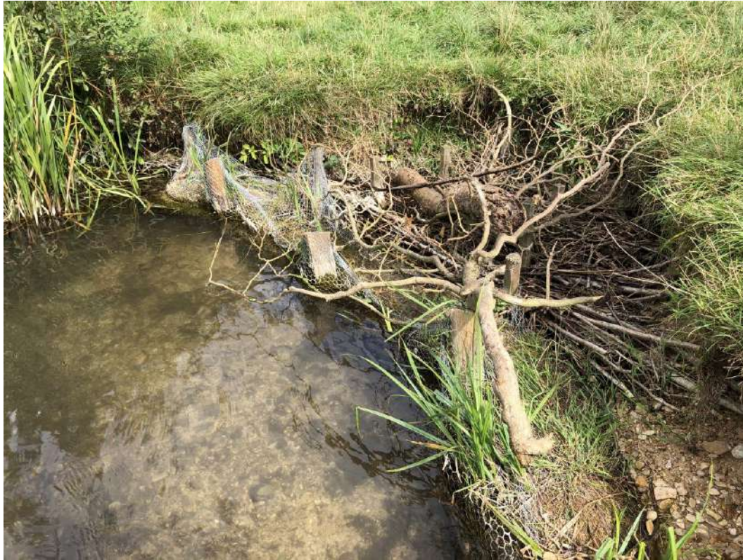
Damaged coir fibre roll installed in front of eroded bank at 11a
